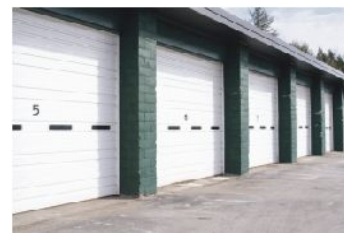
Garages / Overhead Doors
